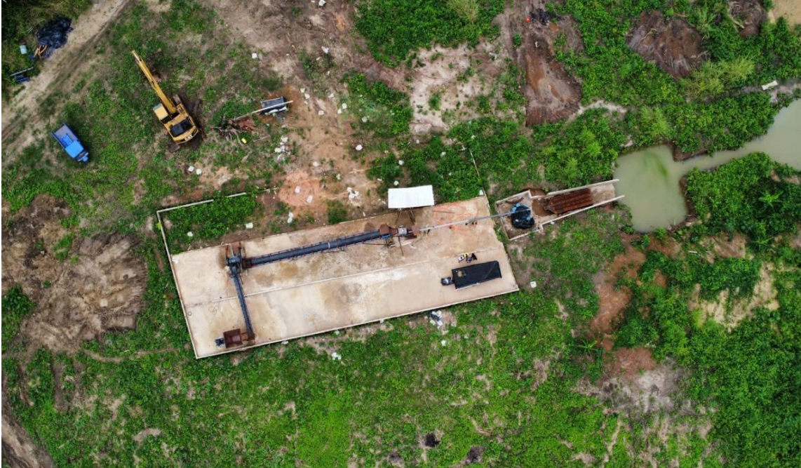
Early construction of the eventual hard rock crushing and sluicing circuit on GFX's current site, November 2023.
